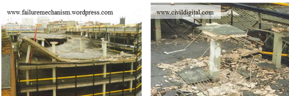
Fig 1-2. Failure of slab-column connections due to punching shear
