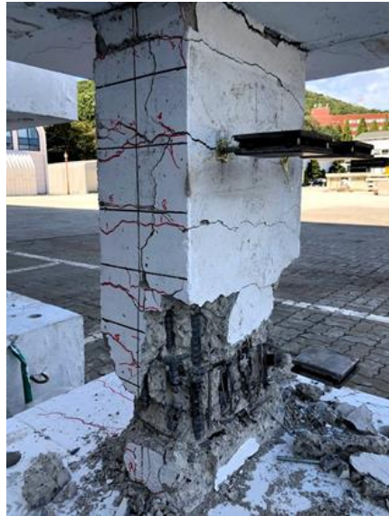
(b) Failure mode
