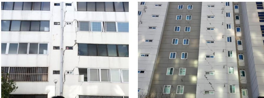
Figure 1-2 Damages of the earthquake in Gyeongju and Pohang
