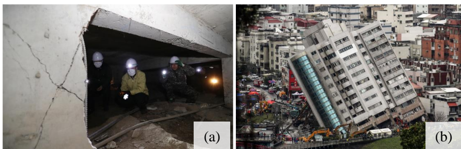
Figure 1.1 Cases of substructure failure: (a) shear failure of columns in the substructure induced by Pohang earthquake in 2017 and (b) substructure failure by Hualien earthquake in 2018
