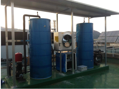
(a) Storage System(전면)
