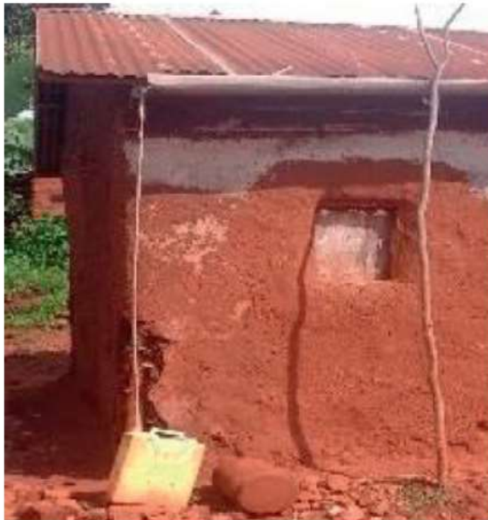
Figure 3. Plastic jerrycan of 20 liters with it dimension used as roof rainwater harvesting storage In Nigeria (Bernard and Joyfred, 2020)
