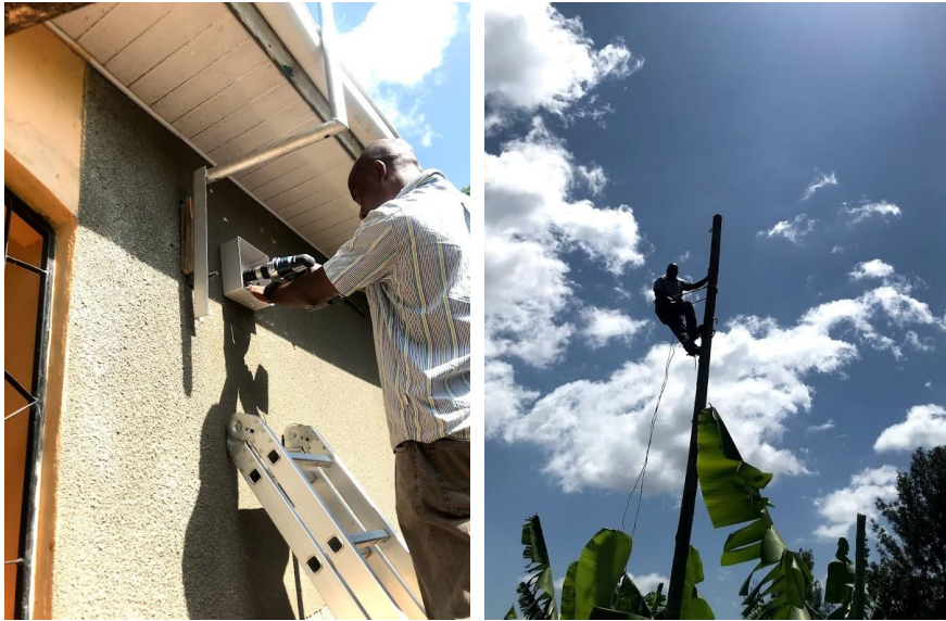
Figure 11. Technician who is installing a SNU-meter on (a) a wall and (b) a pole in Ngurdoto village
