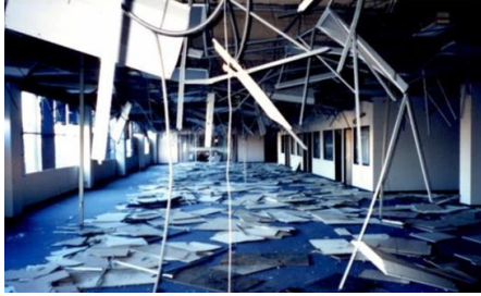
(a) 1994 Northridge earthquake ( M_w = 6.7 )
