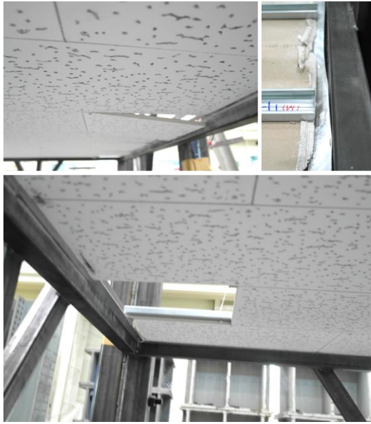
Figure 5.26 Failure pattern of IMC-L-M specimen observed during shake table test
