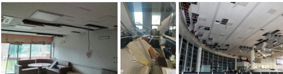
Figure 1.1 Failure of suspended ceilings observed in Gyeongju ( M_w = 5.5 ) and Pohang ( M_w = 5.4 ) earthquakes in Korea.
