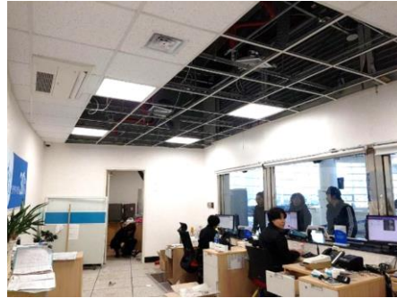
(b) 2017 Pohang earthquake ( M_w = 5.4 )
