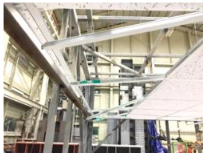
(c) Failure of latch connections
