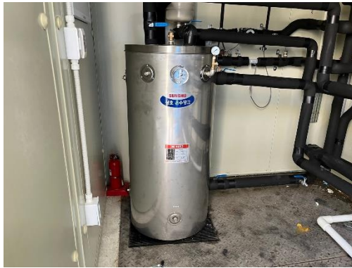
Figure 3.6 Storage tank and the specification
