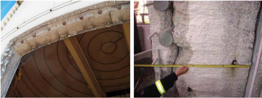
Figure 1-4 Delamination of containment wall at Crystal River (Nuclear Regulatory Commission, (2010))
