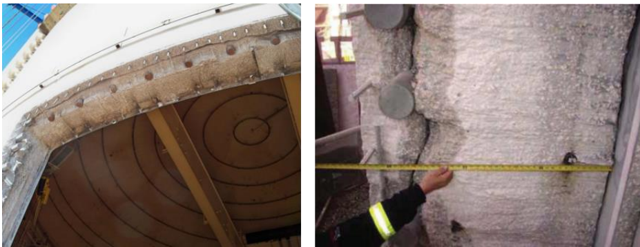
Figure 2-12 Wall delamination at the Crystal River Nuclear Power Plant Unit-3 (Nuclear Regulatory Commission (2010))
