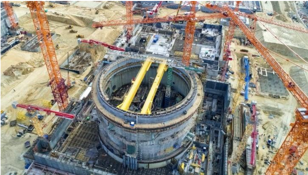
Figure 7-8 A polar crane of containment building
