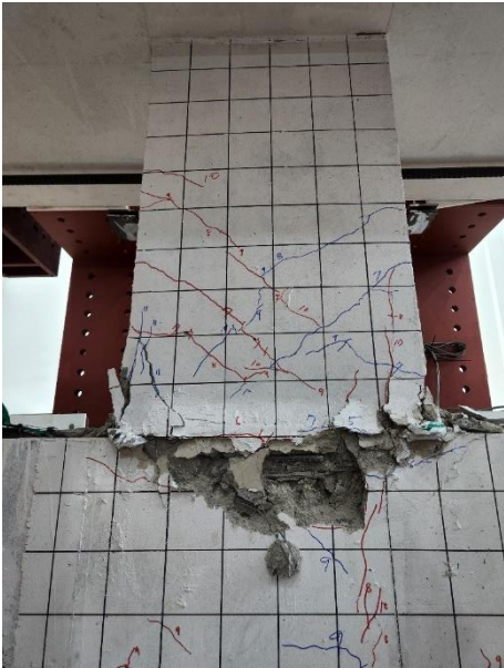
(b) Flexural failure of wall
