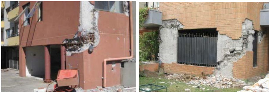
Figure 1-3 Earthquake damage for geometric wall discontinuity
