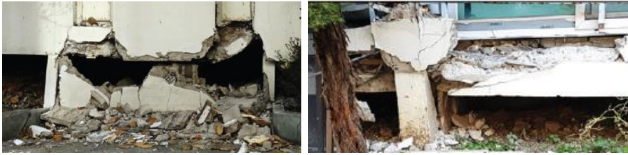
Figure 1-2 Shear failure of Apartment
