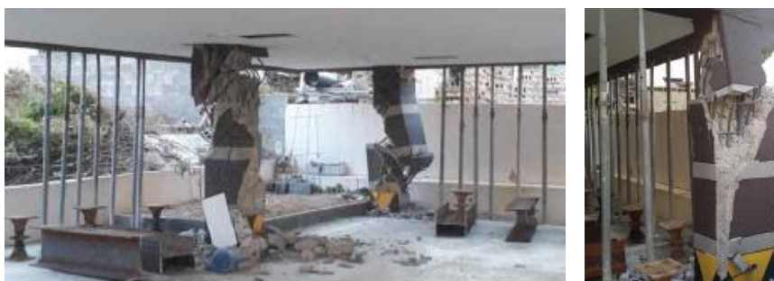
Figure 1-1 Shear failure of Piloti Structure
