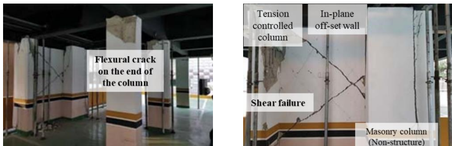
Figure 2-4 Damage in low-rise piloti structure
