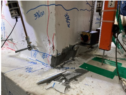
(a) Grout cover delamination ( \delta = 1.5\% )
