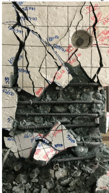
(e) Final failure (front) ( \delta = 6.0\% )
