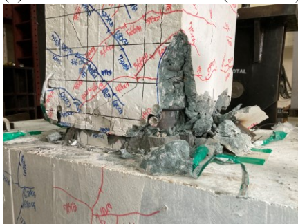
(c) Sleeve cover spalling of a tensile side ( \delta = 4.5\% )
