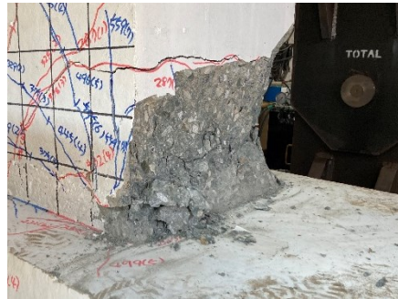
(b) Concrete cover spalling of a compressive side ( \delta = 2.75\% )
