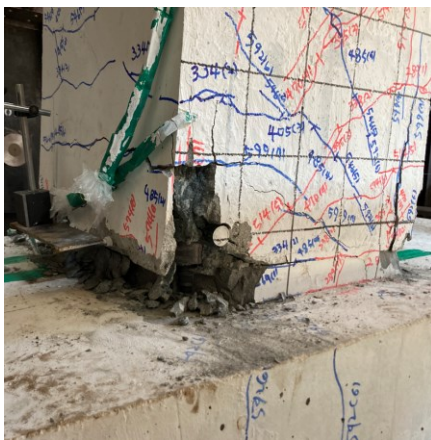
(c) Sleeve cover spalling of a tensile side ( \delta = 2.75\% )
