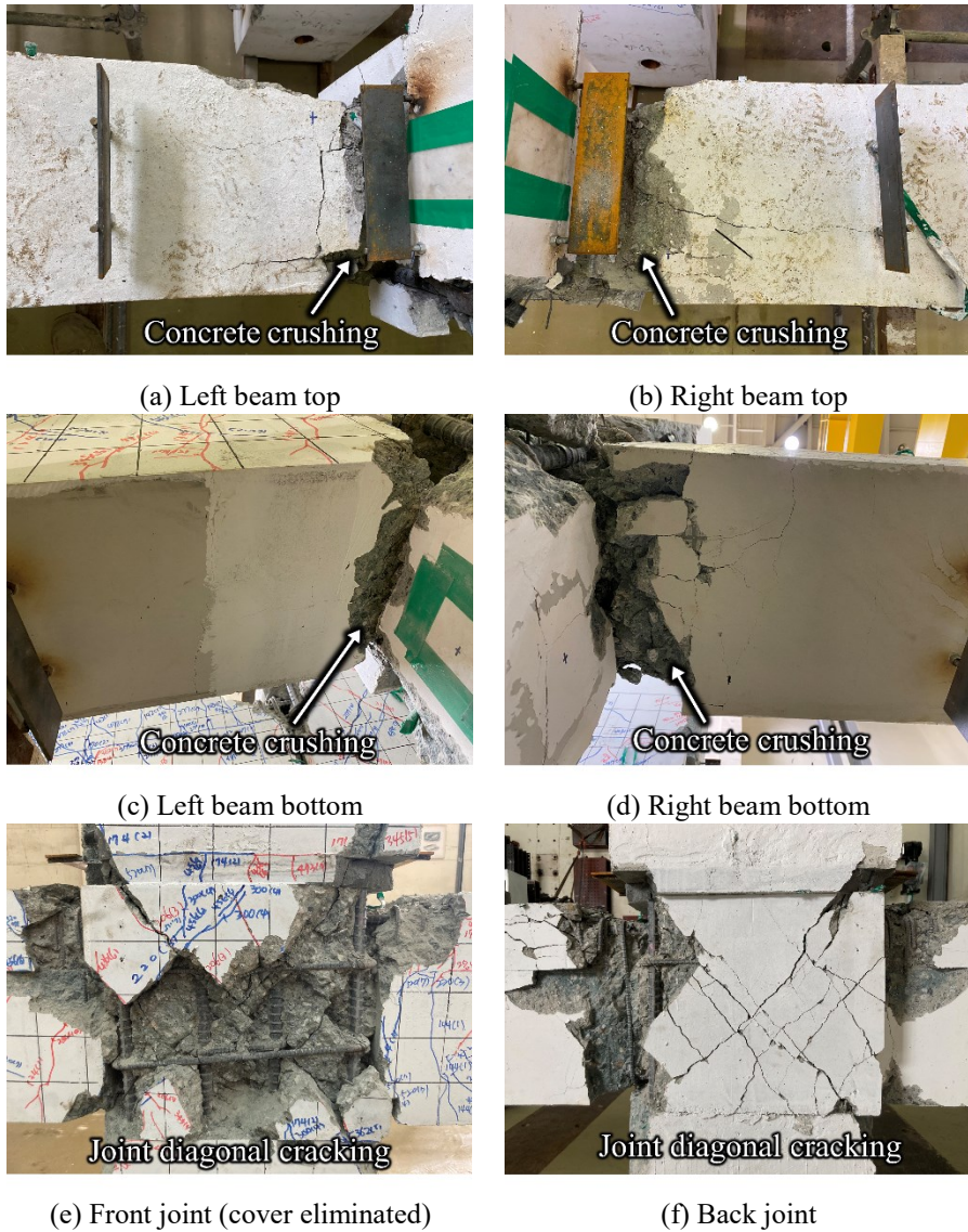
Figure 5-16 J-G2 detailed failure pictures
