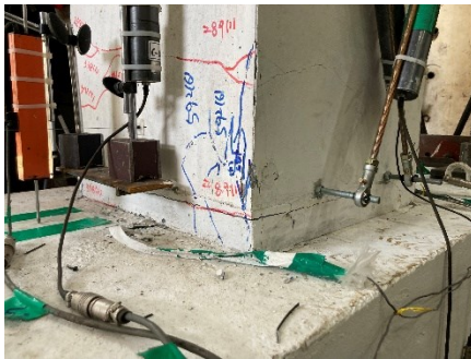
(a) Concrete cover cracking ( \delta = 2.0\% )
