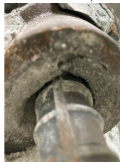
(f) Grout failure inside a sleeve
