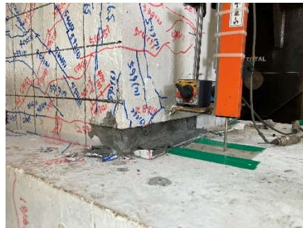
(b) Grout cover delamination ( \delta = 2.0\% )
