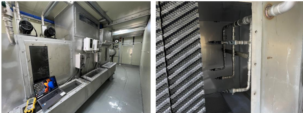
(a) Wet scrubber module with the recirculation pump (b) Washing nozzles inside the wet scrubber module
