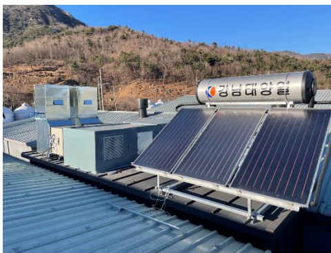
(a) Solar collector and solar water storage tank
