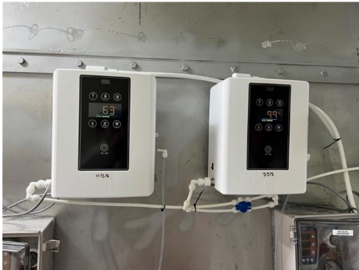
(a) Circulating water treatment device for injecting SAEW
