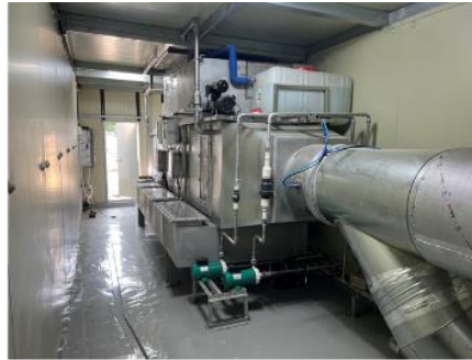
(b) Wet scrubber module connected by duct
