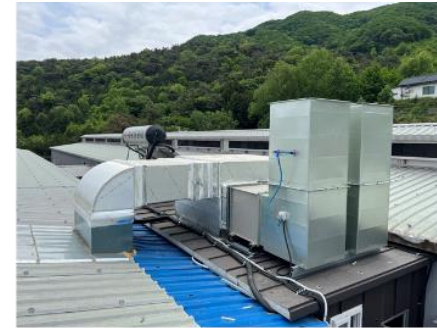
(c) External air mixing module after cleaning
