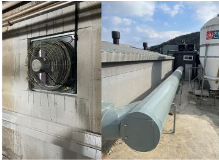
(a) Outlet of piglet room and exhaust duct
