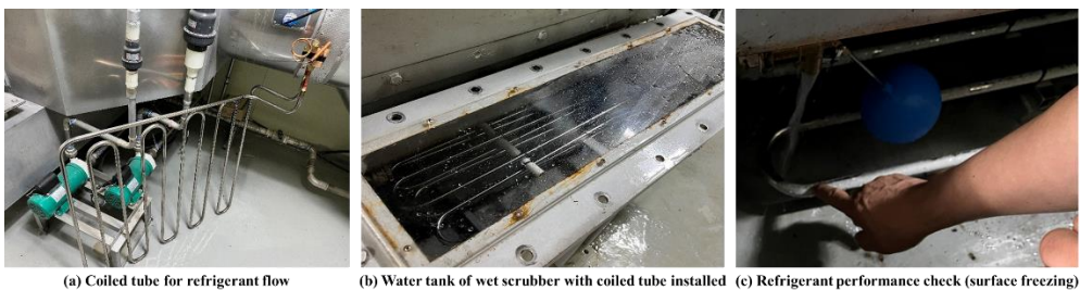
Figure 6-1 Evaporative cooling method using low temperature of the cleaning water using chiller.
